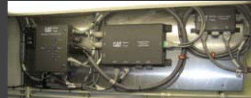
Each Cat Multi-Station Control System supplied is uniquely configured for ease of installation by incorporating plug-and-run components and harnesses made to length. Shown here is the MSCS for the William T.R. as installed by Hike.
