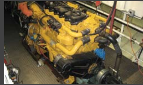
The William T.R.'s customized C18 package allowed for re-use of all existing hydraulic system components along with mounting feet designed for ease of installation.
