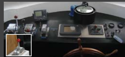
Conversion of William T.R.'s propulsion engine controls include a new Cat single control lever complete with backup controls. The single control lever controls engine speed, gearbox shift engagement, as well as trolling.
