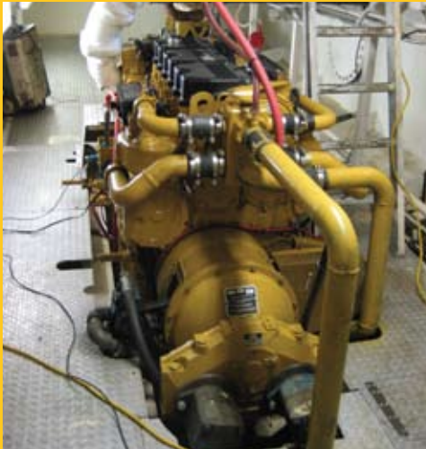
The C18 engine for the Francesca Madre also included a Cat front pump-drive adapter along with Twin Disc's AM220 dual SAE 'C' power take-off. With this equipment package we were able to retain all existing hydraulic pumps onboard.
