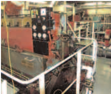
▲ Starboard and port Caterpillar MaK 6M20 propulsion engines each rated 1550bhp at 1000rpm provide “M/V Jiimaan” with 12kts at 85% CSR. Note ease of access to the cylinder heads and cylinder block. All fluid filter elements are cleanable to eliminate disposal costs.
